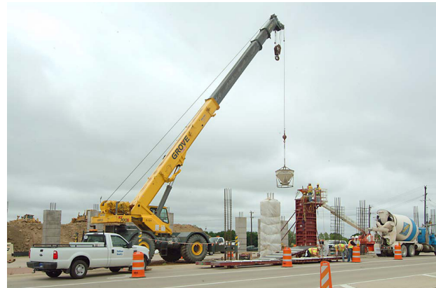
Major improvements to the Dallas North Tollway won Project of the Year honors from the Texas Chapter of the American Public Works Association, bestowed in 2005.
